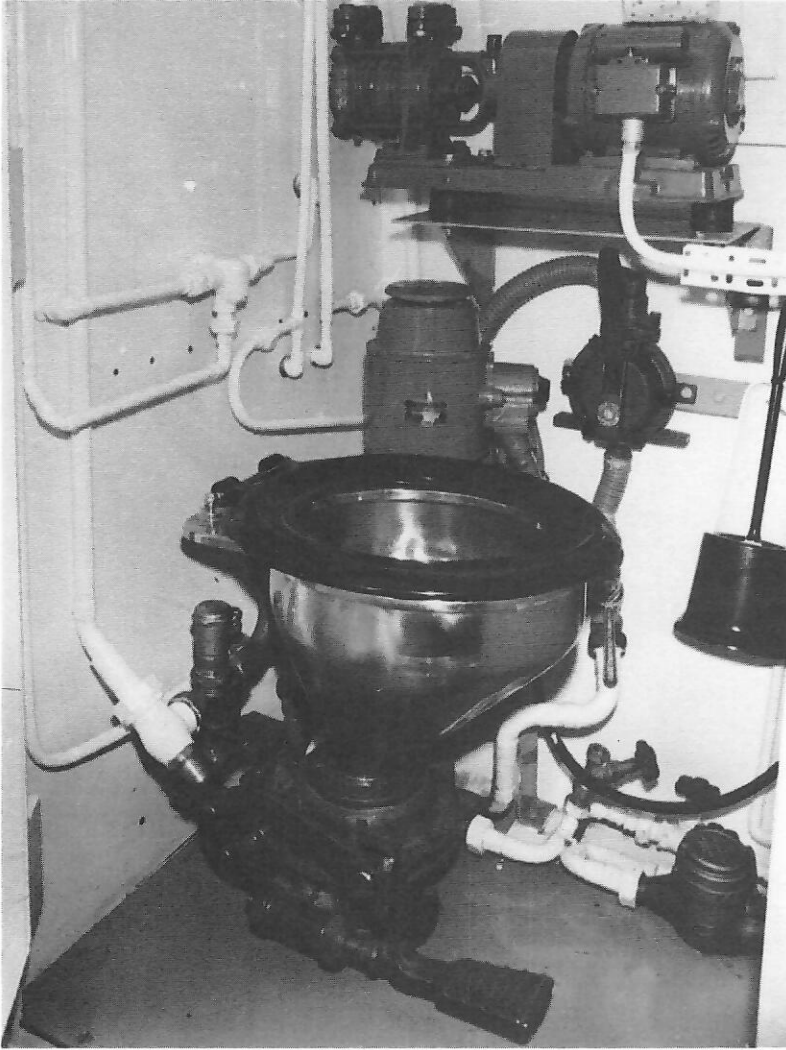
Fig. 6.46. WC compartment with water lavatory, water pumps and control valves on the under-water laboratory Helgoland .
