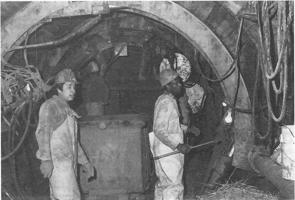
FIG. 1.3. Workmen at the face of an 8 ft (2.4 m) finished bore sewer tunnel being driven under 43 psig (394 kPa) pressure. The tunnel lining is made up of 4 ft sections of maple heart timbers supported by steel ribs. The straw is used for caulking the invert. Hydraulic fluid, straw and wooden planking present serious fire hazards. (Courtesy of Wisconsin Department of Health)
